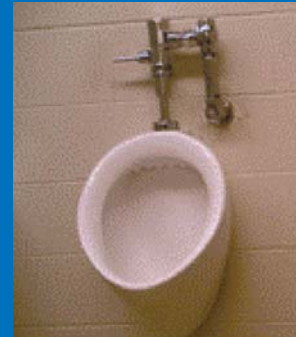
University of Washington: Non-Zurn 0.5 GPF urinal system. Notice the alter- ations made in the pip- ing in order to fit the footprint.
